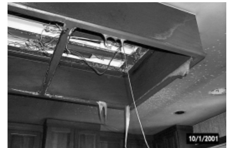
Intense heat melted the plastic cover on the fluorescent light fixture over the range top.
