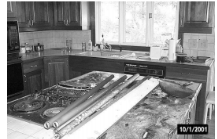
This residential fire began when meat was left cooking unattended on the range top.
