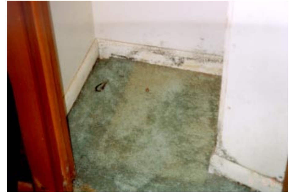
Mold infested carpet and pad are porous materials and should be removed and replaced
