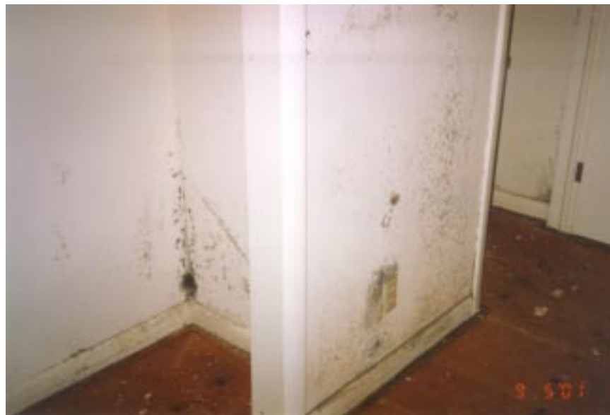
Removal of mold infested materials can cause health problems
