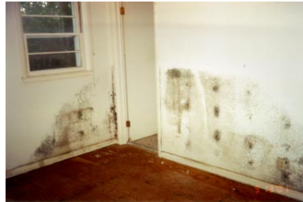
Visible mold colonization on drywall
