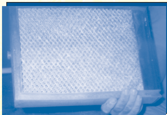
HVAC filter contaminated by excessive pollen.
