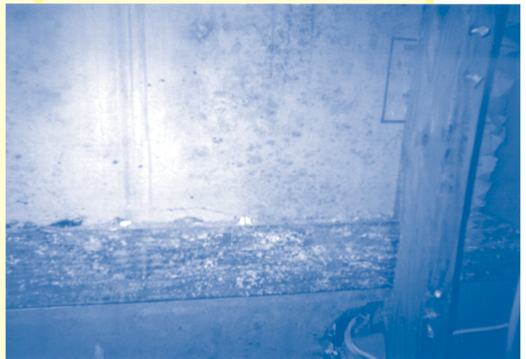
Mold growth inside wall cavities.
