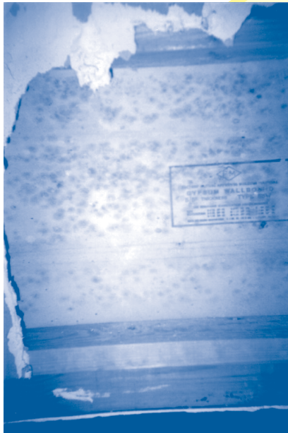
Previously installed sheetrock had to be torn away to reveal mold inside.
