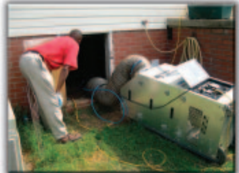
The HEPA vacuum is attached to the heating system under the house.
