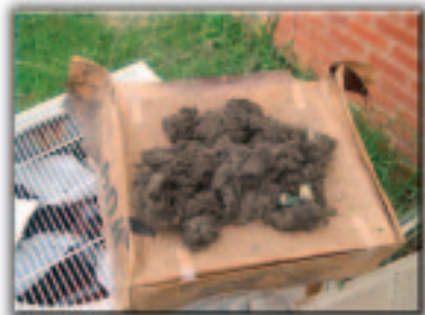
Some of the ??? dust & dirt removed from the ductwork during cleaning.
