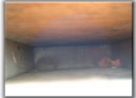
Debris & greasy dust block airflow inside the kitchen register.
